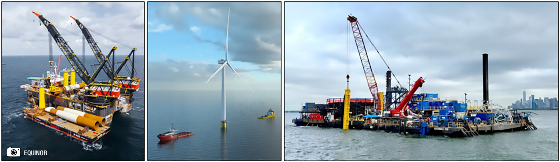
Figure 16: Monopile installation using a semi-submersible crane vessel, driving the piles to sub-seafloor depths of 50 m (left). Installed 15 MW turbines with a rotor diameter of 260 m, with tips reaching 290 m above sea level (middle). Cable laying along the 75 km route from south Brooklyn to the offshore substation (right).
